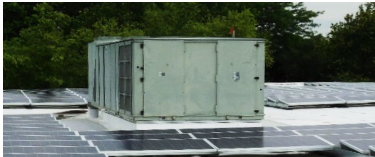
An example of a large piece of rooftop equipment adjacent to PV modules. (Source: ZRS)
